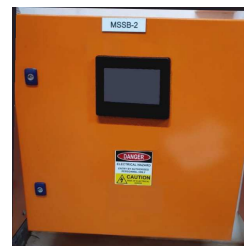
Typical wall-mounted installation for small apartment block.
